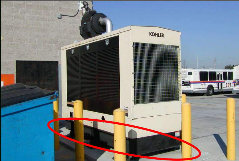
Bulk storage container (stationary AST)
