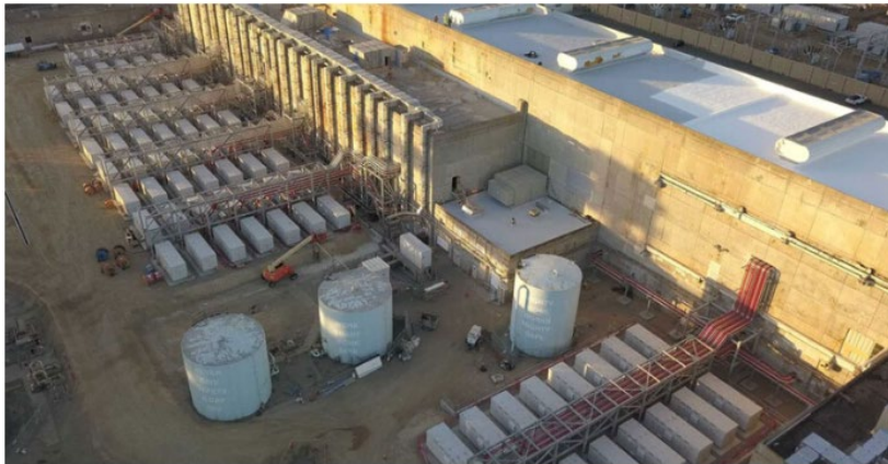
Moss Landing Energy Storage Facility
