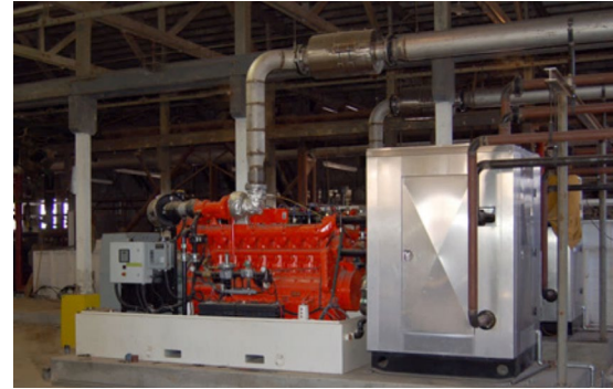
A large industrial application
