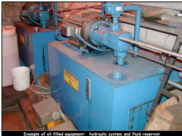
Example of oil filled equipment: hydraulic system and fluid reservoir
