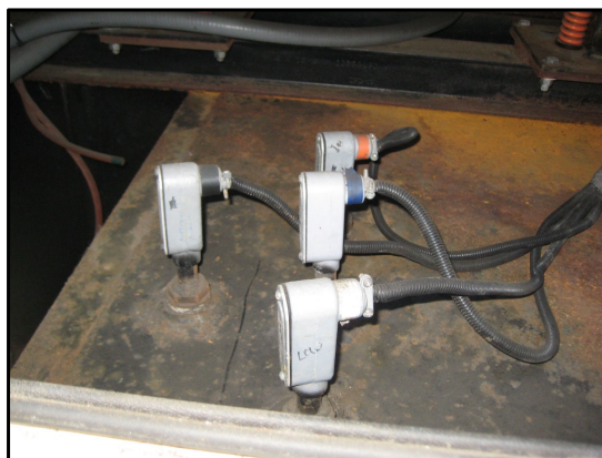
Interstitial leak sensor at left, with low, high, and high-high level sensors at right
