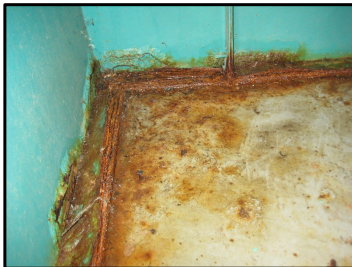
Corrosion of tank top surface and enclosure sides from standing water
