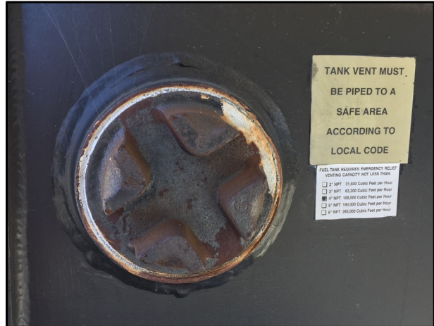
Steel plug on emergency vent on generator base tank
