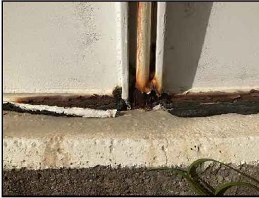
031 Active Corrosion on Anchor Chair X
