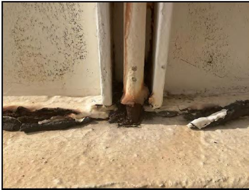
033 Active Corrosion on Anchor Chair Z
